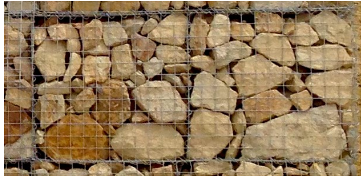
Above (Option 2): Gabion wall at neighborhood monument. Rotate stones when placing in basket so face of stone is flat to basket, minimizing voids along face of wall.
